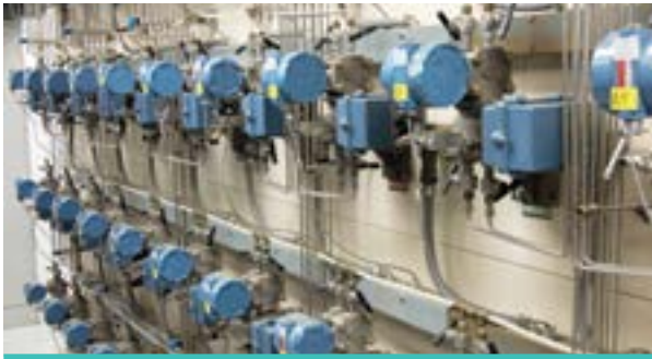
BWXT's data acquisition system includes a wide variety of instrumentation, as well as the capability to provide live data during testing.
