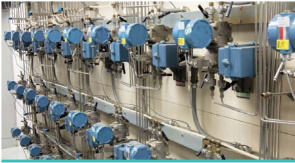
BWXT's data acquisition system includes a wide variety of instrumentation, as well as the capability to provide live data during testing.
