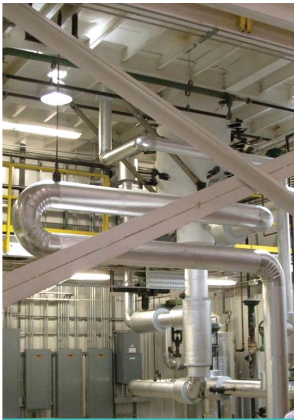
BWXT's test facility contains a number of flow loops with flexibility to configure components for each customer's unique requirements.
