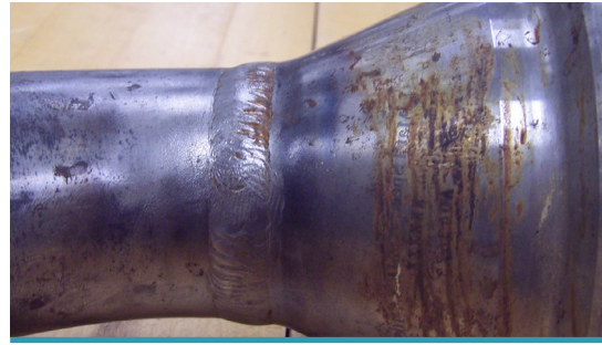
CANDU feeder tube Grayloc weld region
